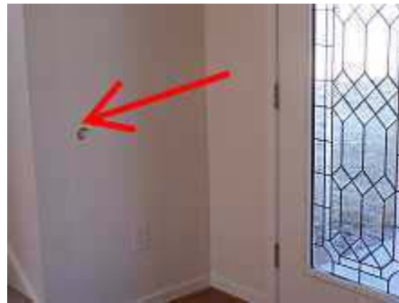
Photo 38 Hole in wall from front door. No door stopper installed.
