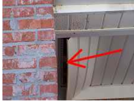
Photo 24 Siding coming loose on front porch.
